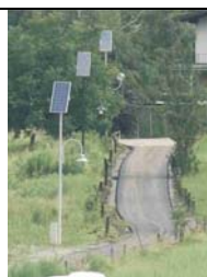
Plate 3: The unsurfaced path leading from the Vorarlberger Medienhaus to the station was unattractive in bad weather and was therefore surfaced with asphalt. The staff's frequently expressed wish for lighting was met in an innovative and environmentally friendly way (solar-lighting masts).
