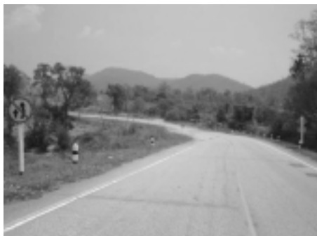
Highway 106 km. 29+410-29+470 (Lampoon - Lee): Sharp curve on mountainous area without chevron signs and insufficient roadway markings.
